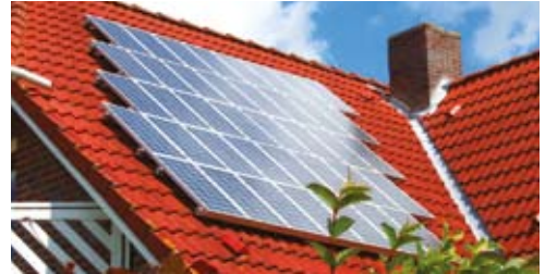
Photovoltaic Solar Collectors
